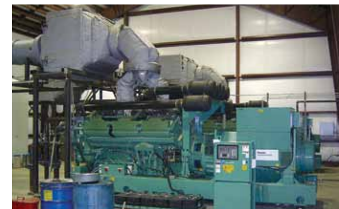
Engines used in power generation.
